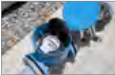
Discharge to Sewer Flow Meters
